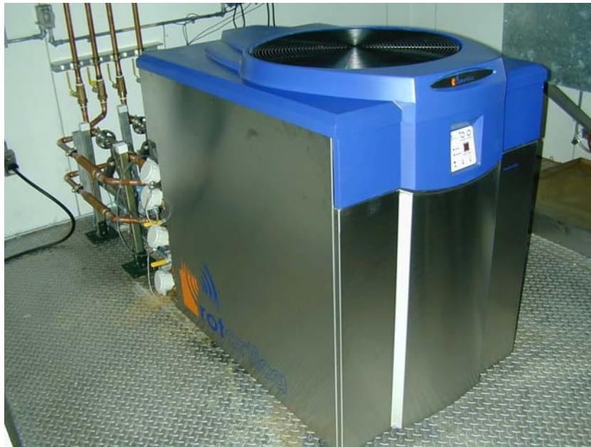
Figure 3. Picture of RAC unit.
