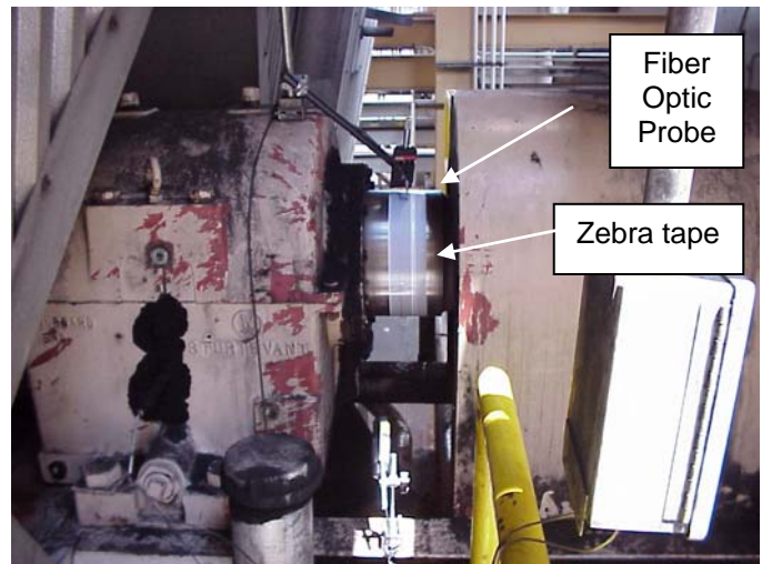
Figure 2D. Zebra tape encoder and fiber optic transducer in limited rotating shaft access installation.
