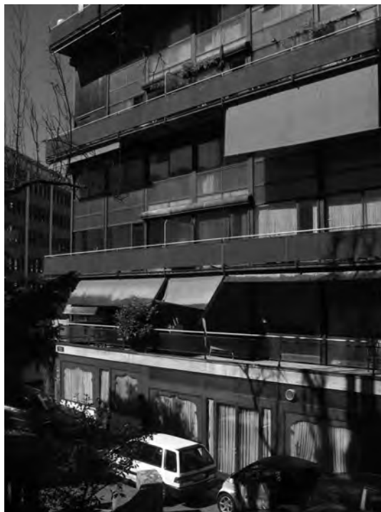
Figure 7: Immeuble Clarté, south façade with balconies, awnings, and wooden screens (photograph by author).
